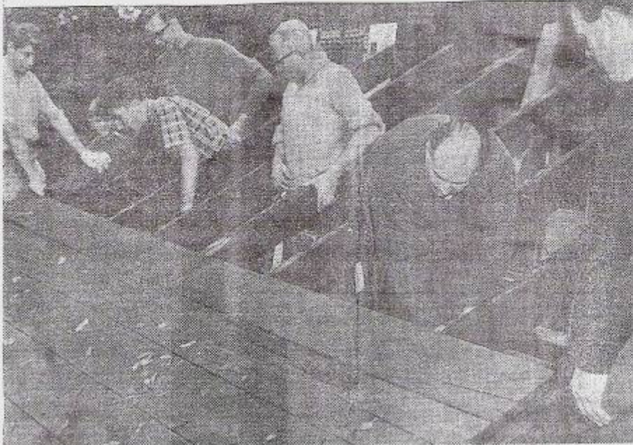
Work is now well under way on the new headquarters being built for the ninth Greenford (Holy Cross) Scout Group behind Holy Cross Church. The floor has been laid and parents and friends are now preparing to erect the walls. It is hoped that the building will be up by November
